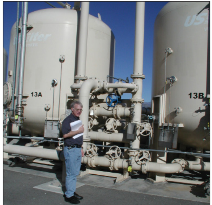
Conducting a site inspection of the treatment plant at the Newmark Ground Water Contamination Superfund Site in San Bernardino, California.
